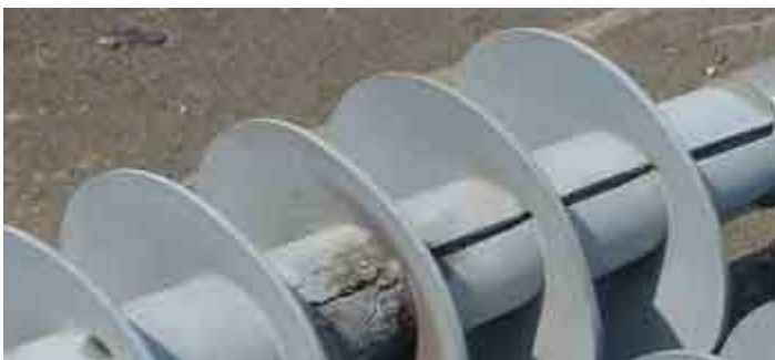
Fig.1: NCI Line Post that was removed from service in Southern USA
