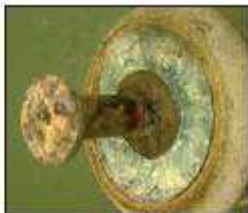
Figure 2 Shattered glass insulator with corroded pin
