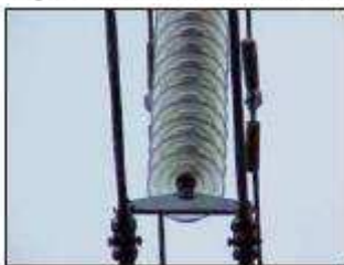
Figure 5 Glass insulator string
