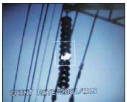
Figure 8 Corona caused by adjacent faulty insulators
